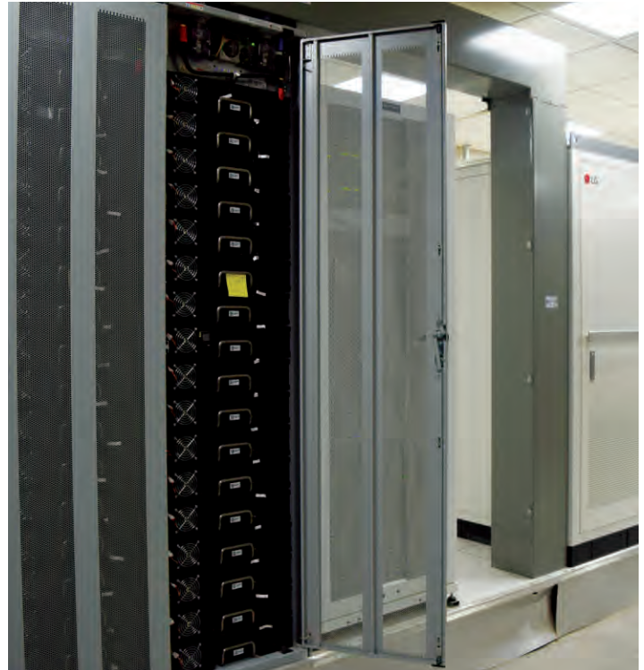
The LG Energy Storage System (ESS) in the Sinclair Hotel basement is now the first lithium-ion battery system in the world to be used as a replacement for the required backup diesel generator. It’s also UL 924 rated and provides peak load shaving in the building.
