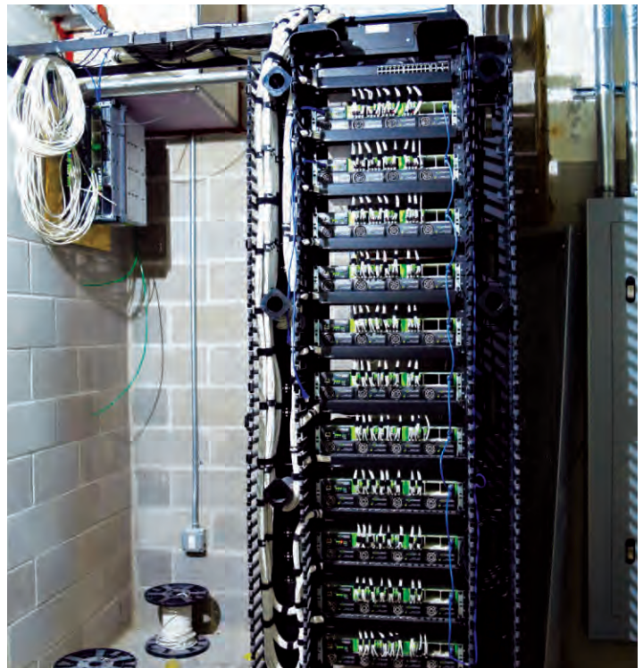
Superior Essex cable acts as the backbone for transporting power up from the basement to these IDF closets on each of the hotel’s 16 floors.
