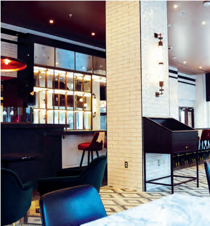
There are over 5,000 lights installed throughout the hotel, as seen here in the hotel restaurant and lobby bar, each powered and connected to the network with PoE cable.
