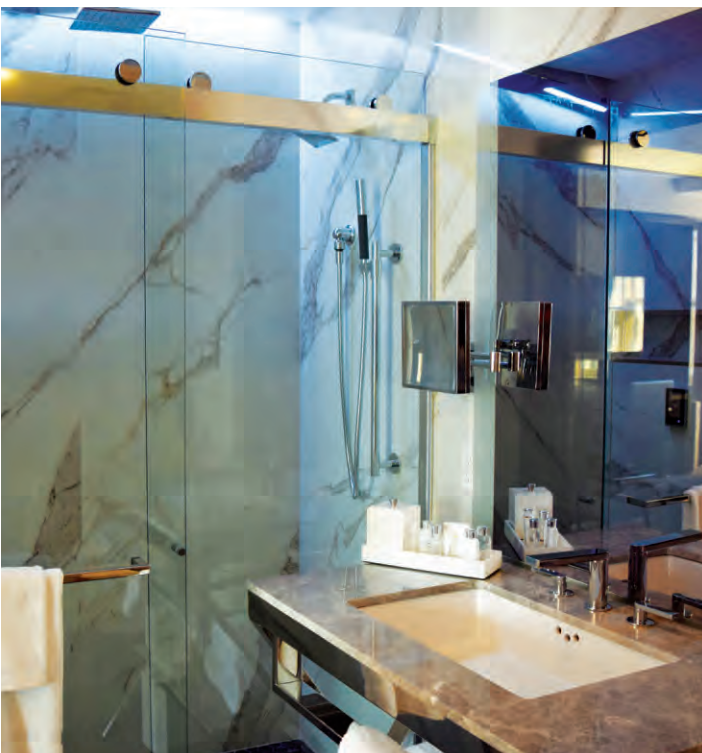
The hotel suites, with their gorgeous amenities and fixtures, utilize PoE cable to power, connect and control more than 30 devices in each room, including the bathroom lights, electric mirror and even the shower head.
