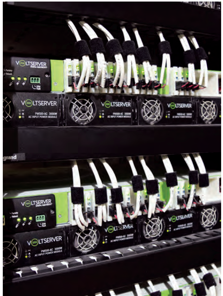
The building’s VoltServer DC power distribution system sends packets of smart “digital electricity” throughout the hotel via over 286,000 feet of Superior Essex PoE cable.
