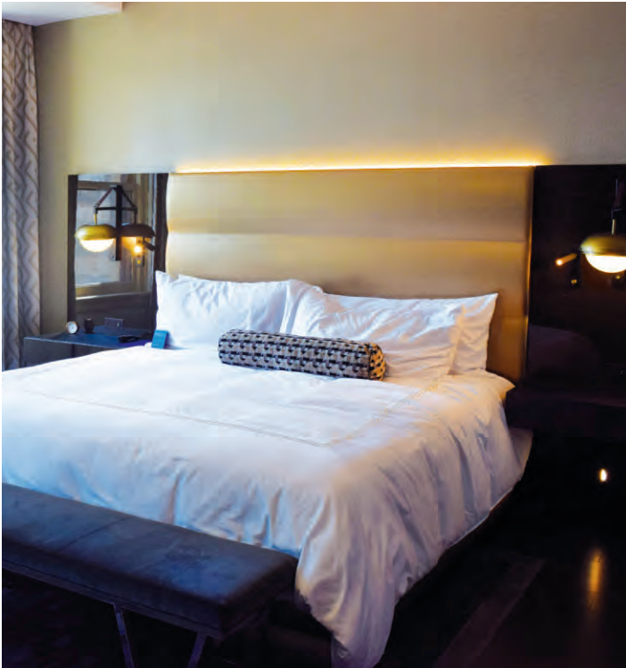
A single Superior Essex 18 gauge/8 conductor PoE cable powers the bed headboards, each of which features seven lights.
